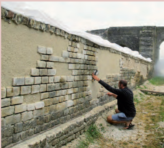
Fig. 123 – City wall. The poor state of preservation of the restoration undertaken more than 100 years ago at the East Gate requires new work to secure and consolidate the masonry.
